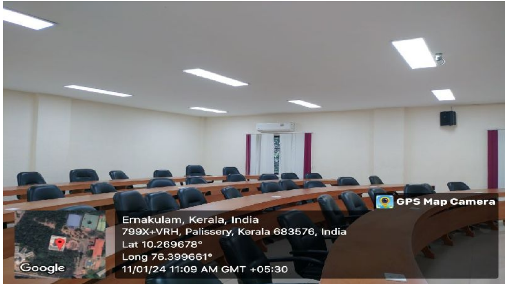
Figure no.9 - Transition to Energy-Efficient LED Lighting
