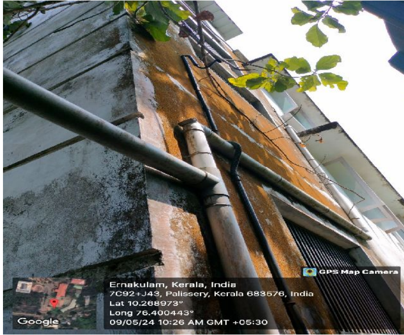
Figure no.2 Collection of rain water from roof tops
